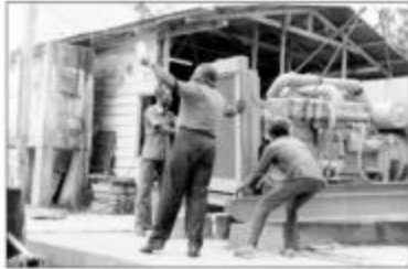
Installation of a New Generating Set at the Power Station, Ikogosi-Odelele , Rivers State.
