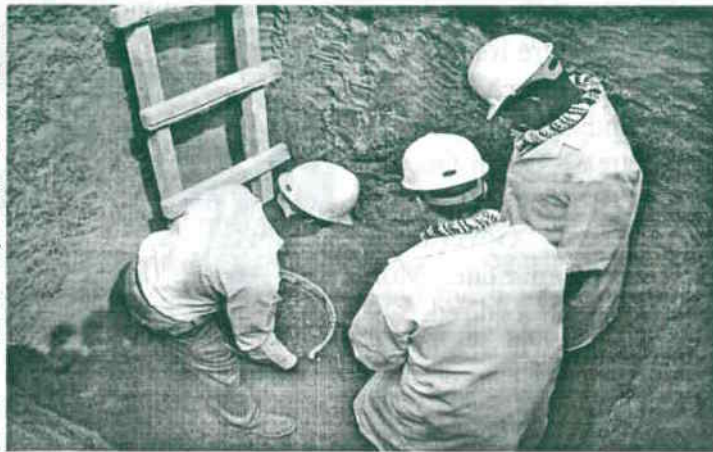
Rev. Darrel D. Lee (middle) lays the first block of the International Worship Centre at Igbesa. With him are Reverends Akazue (right) and Aremu (the project manager)
