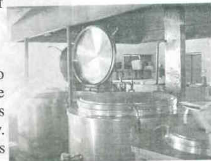
Modern Kitchen Boilers
